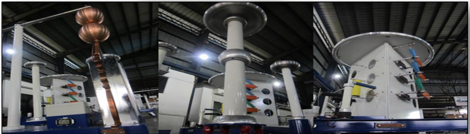
• State-of-the-Art Transformer Testing Facility
